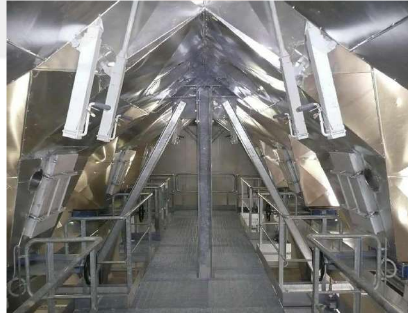
Hoppers arrangement and access
